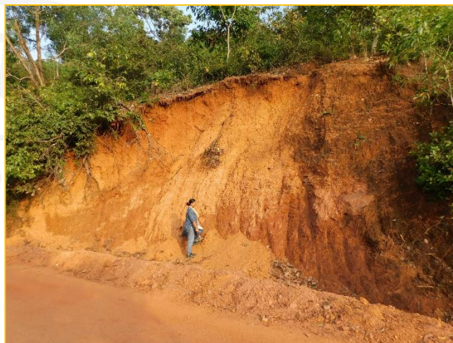
Photo 3. 2a, Slope cut failure near Kodani village Lat: 14° 13' 53.24" Long: 74° 34' 1.88"
