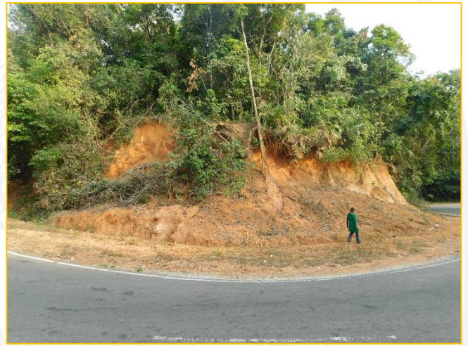
Photo 3. 4b, Soil slide along NH-206 Lat: 14°13' 43.31"Long: 74° 48' 56.64"
